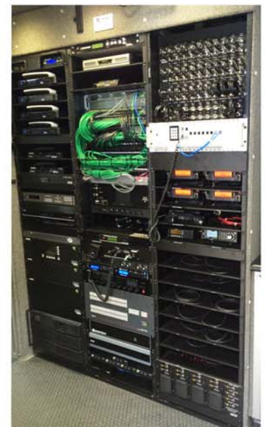
Full-height equipment racks
