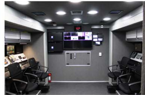
Rear wall Communications Room
